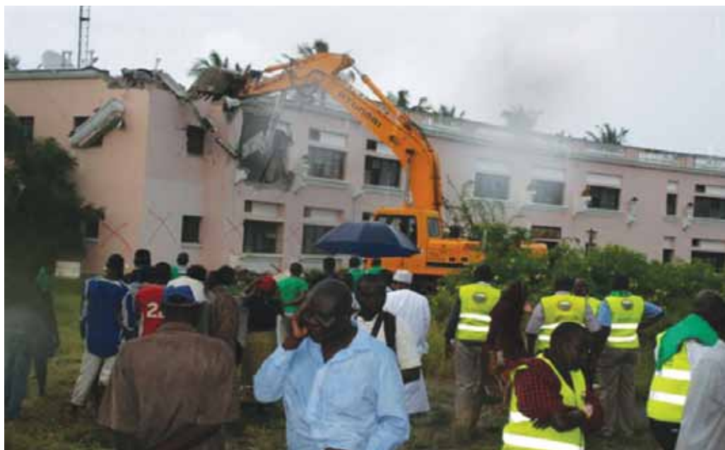
Demolition of the Safari Club Hotel built on a road reserve in Shanzu, Mombasa on 27 th June 2013.
